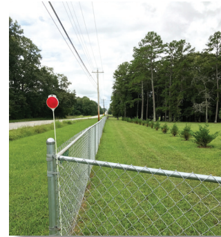
The trees in this photo are planted with the powerlines in mind, when they mature they will not be close enough to touch or create an arc.
