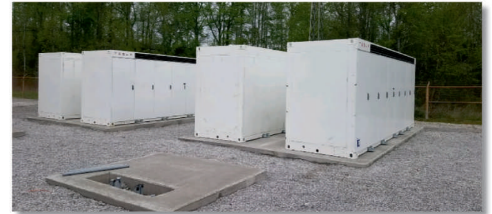
VEC steps into the future of peak and voltage management with four Tesla Megapack BESS.
