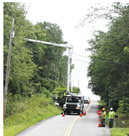
Bucket Trucks and other large equipment are used to remove branches and trees that are in the ROW.
