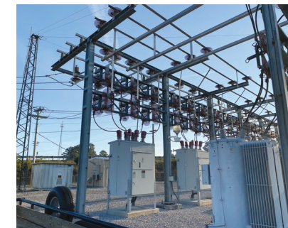
Upgrades in the Ocoee Substation
